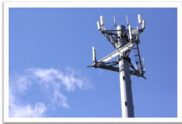
Figure 44 Example of telecommunication facility that could cause frequency interference
