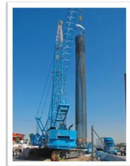
Figure 72 Construction cranes can be considered an obstacle around an airport
